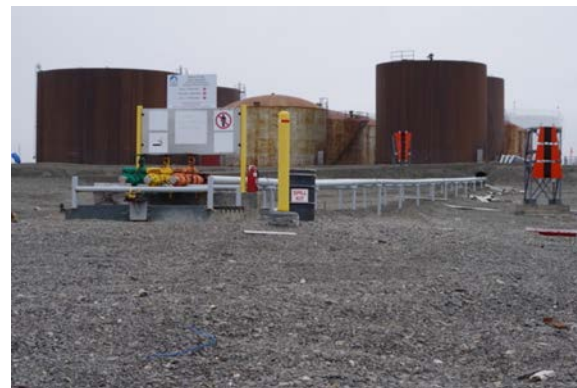
Resolute Bay Oil Handling Facility
